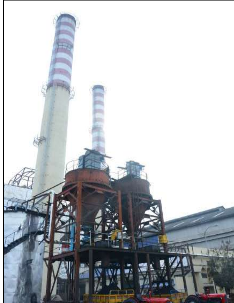
Boiler Ash Handling System
